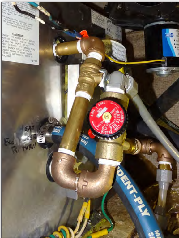
New valve in place - 1
